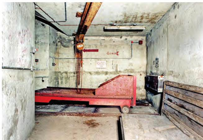
Railed trolley for lowering equipment into the bunker. The trolley ran on rails that straddled the emergency stairs. Photo Nick Catford
